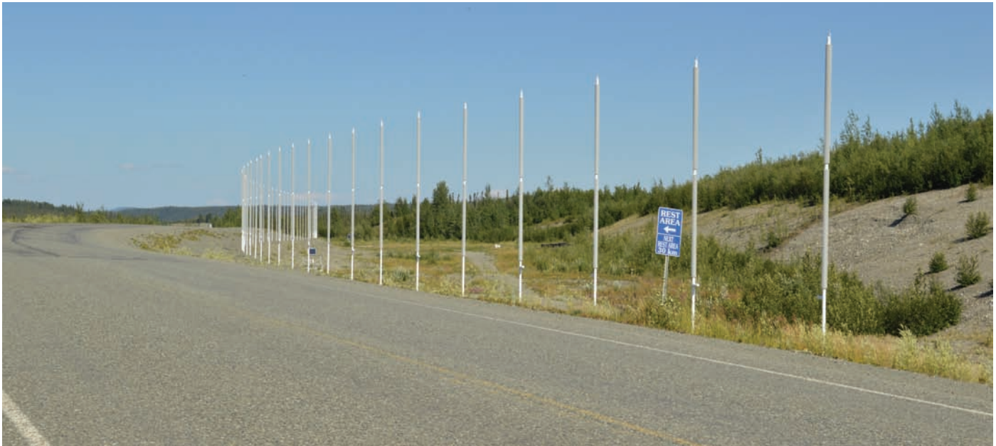
FIG. 12. Thermosyphons installed along the Alaska Highway at Dry Creek, YT (km 1840). These passive ground cooling installations are required to prevent a body of massive ice beneath the road from thawing. Photograph taken on 31 July 2021, © C.R. Burn.
