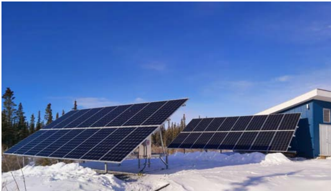
Fig. 1. Recently installed solar panels at the Kluane Lake Research Station. Half the panels are ground mounted (pictured) and half have been placed on the mess hall roof.
