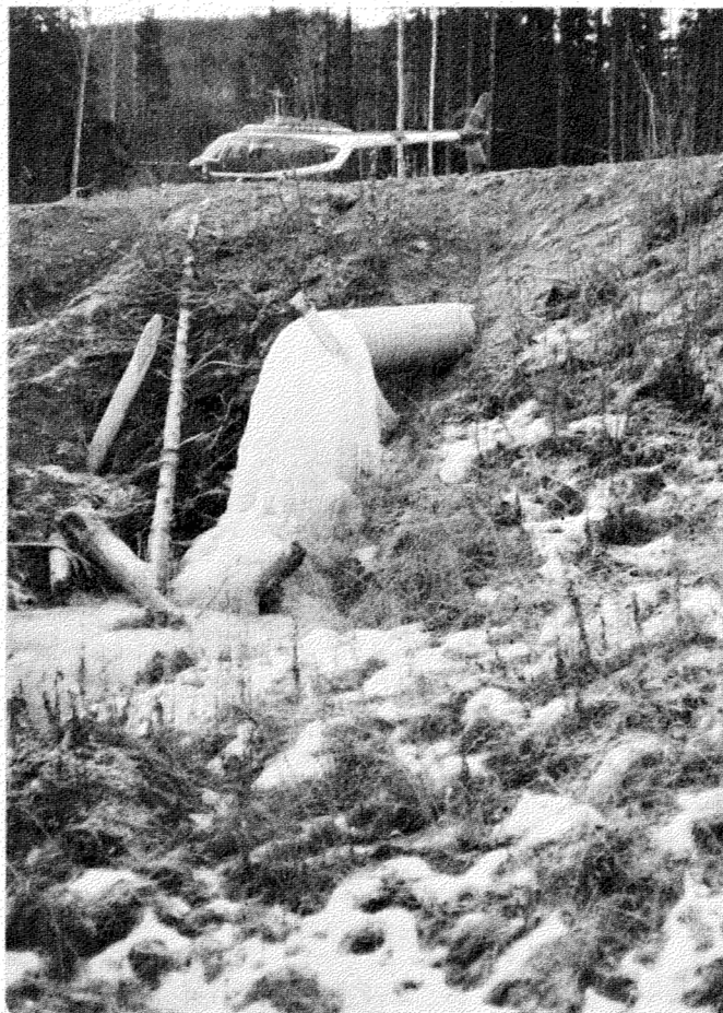
FIG. 9. Culvert blocked by ice, northeastern British Columbia.
