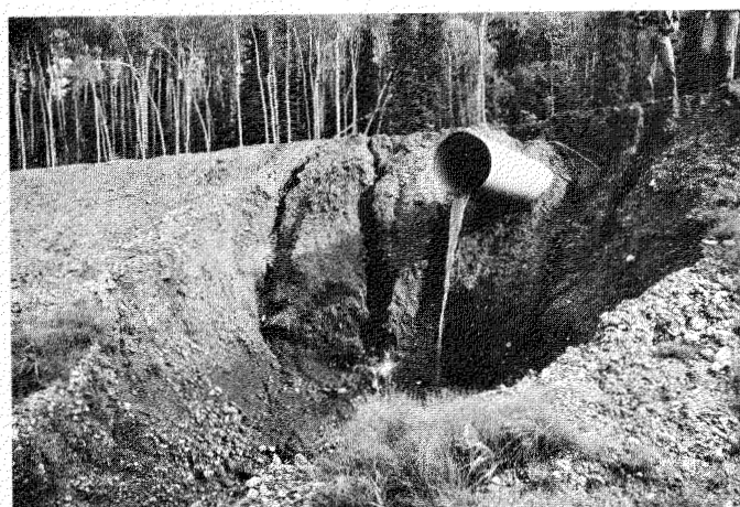
FIG. 7. Erosion below outlet of road culvert due to absence of a let-down structure — Klondike Highway, Yukon Territory, 1978.
