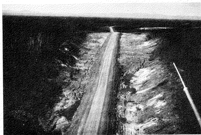
FIG. 2. Cut in ice-rich silty soil — Dempster Highway, Northwest Territories. Location — near Arctic Red River, 1978.
