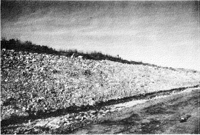
FIG. 12. Blanket of crushed rock protects a road cut from thermal and hydraulic erosion. Cut is located on Dempster Highway, Northwest Territories.
