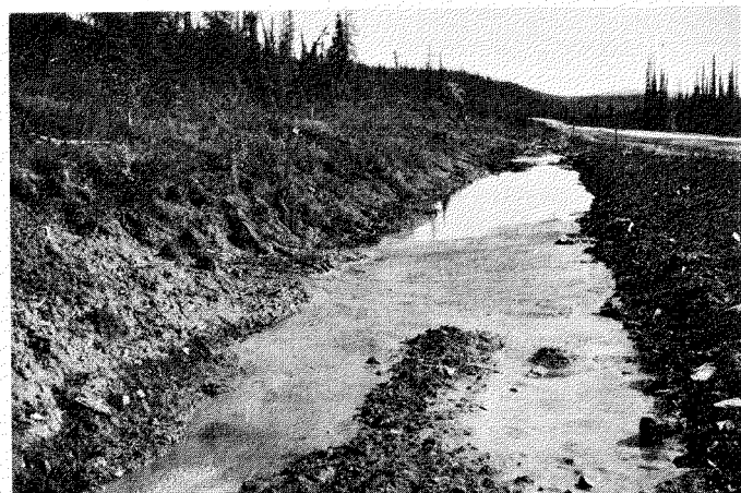
FIG. 3. Ditch slope slumping and regressing — Dempster Highway, near Eagle River, Yukon Territory, 1978.
