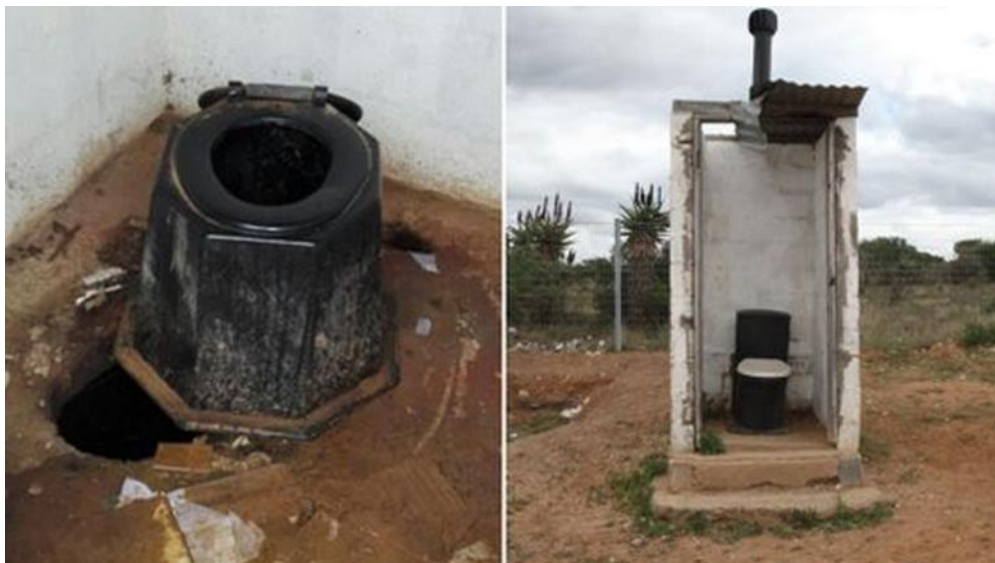
Graphic Evidence of Pit Latrines in South African Schools
